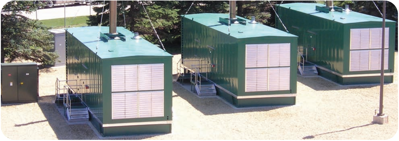
Distributed generators at Austin Utilities
